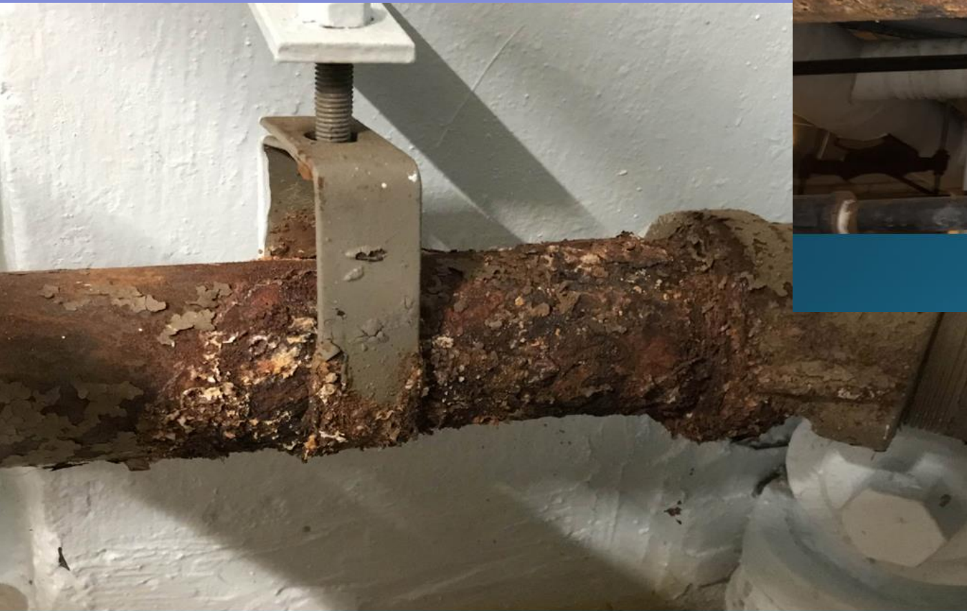
Section of steam heating condensate return piping. Much of piping is original to building: 73 years old.
