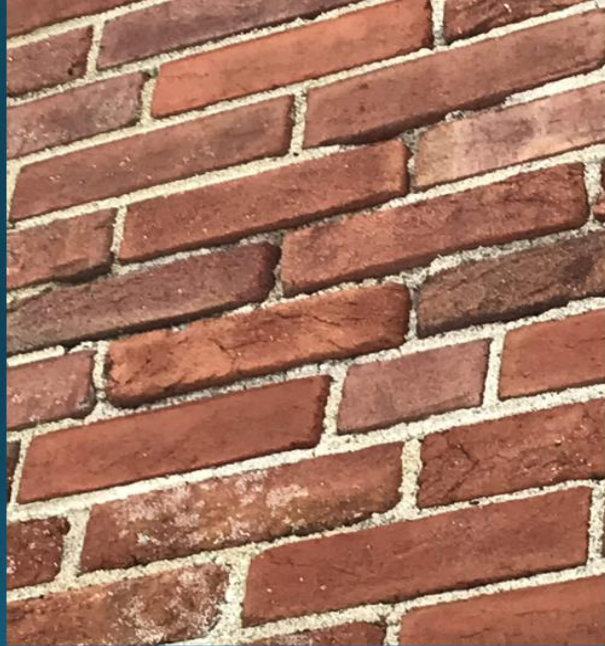
Exterior brick additional repointing needed
