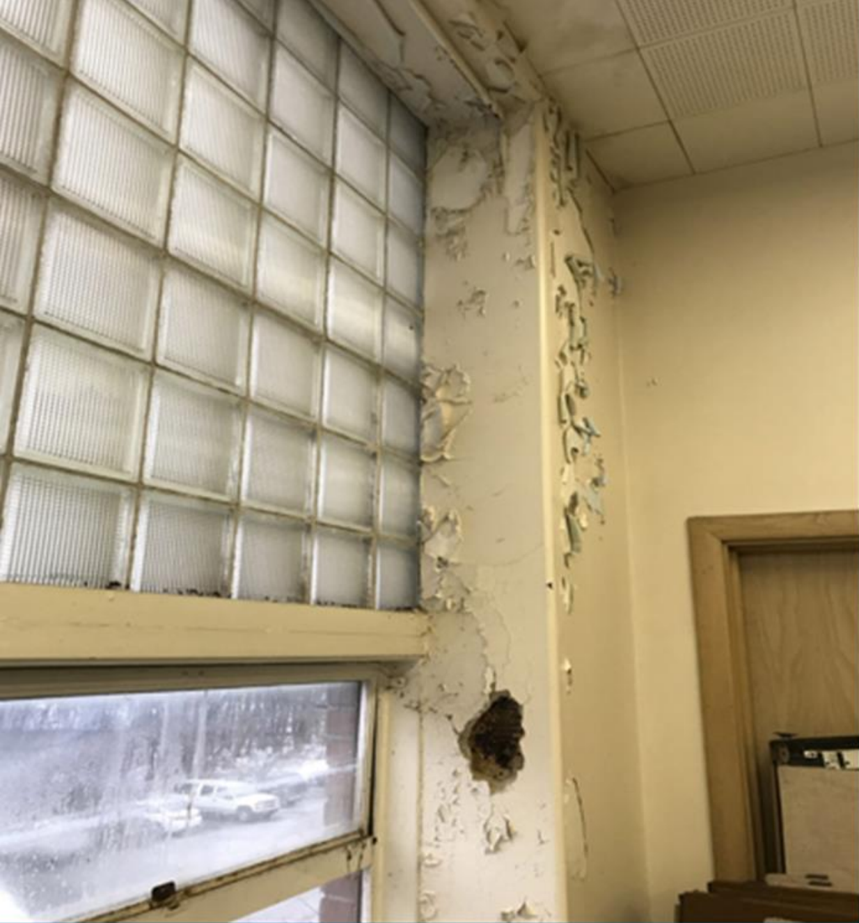
Third Floor paint and plaster condition.
