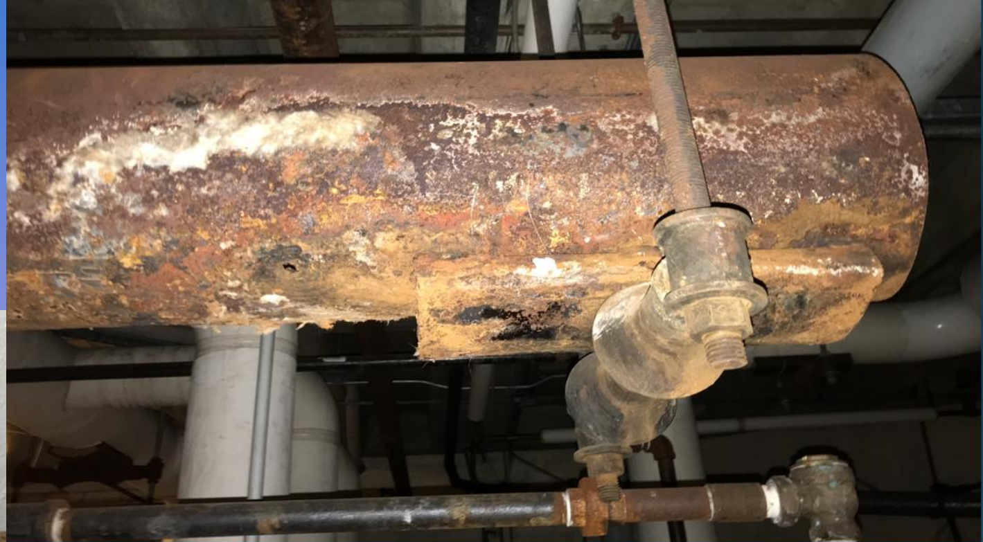
Abandoned section of main steam supply piping: no longer in use for abandoned back-up boiler.
