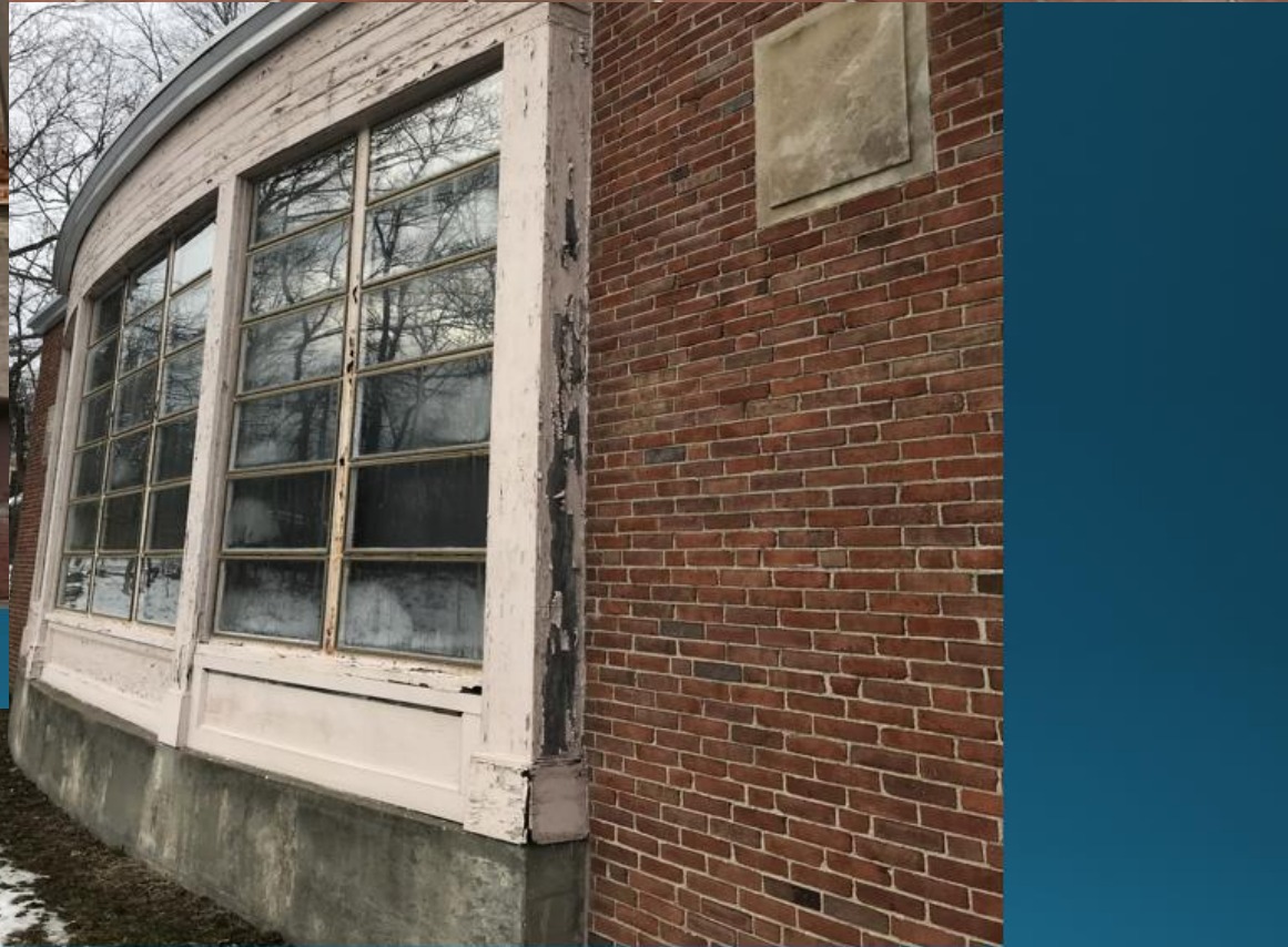
Exterior showing rotted wood trim and condition of steel windows
