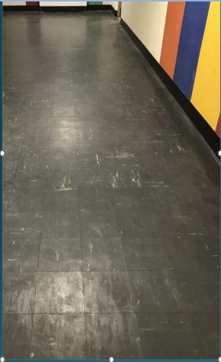
Asbestos-containing floor tile Third floor hallway.
