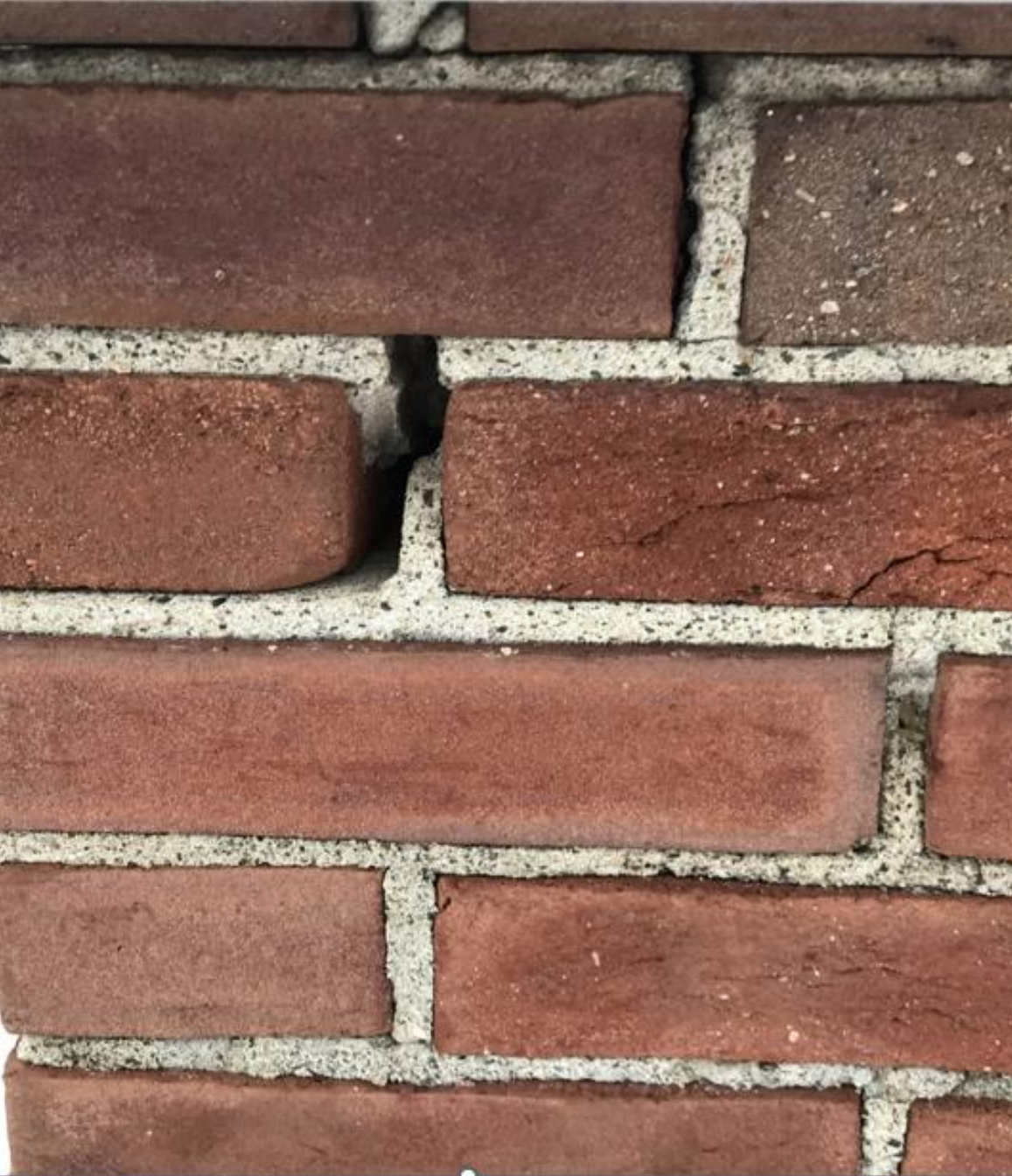
Exterior brick displacement.
