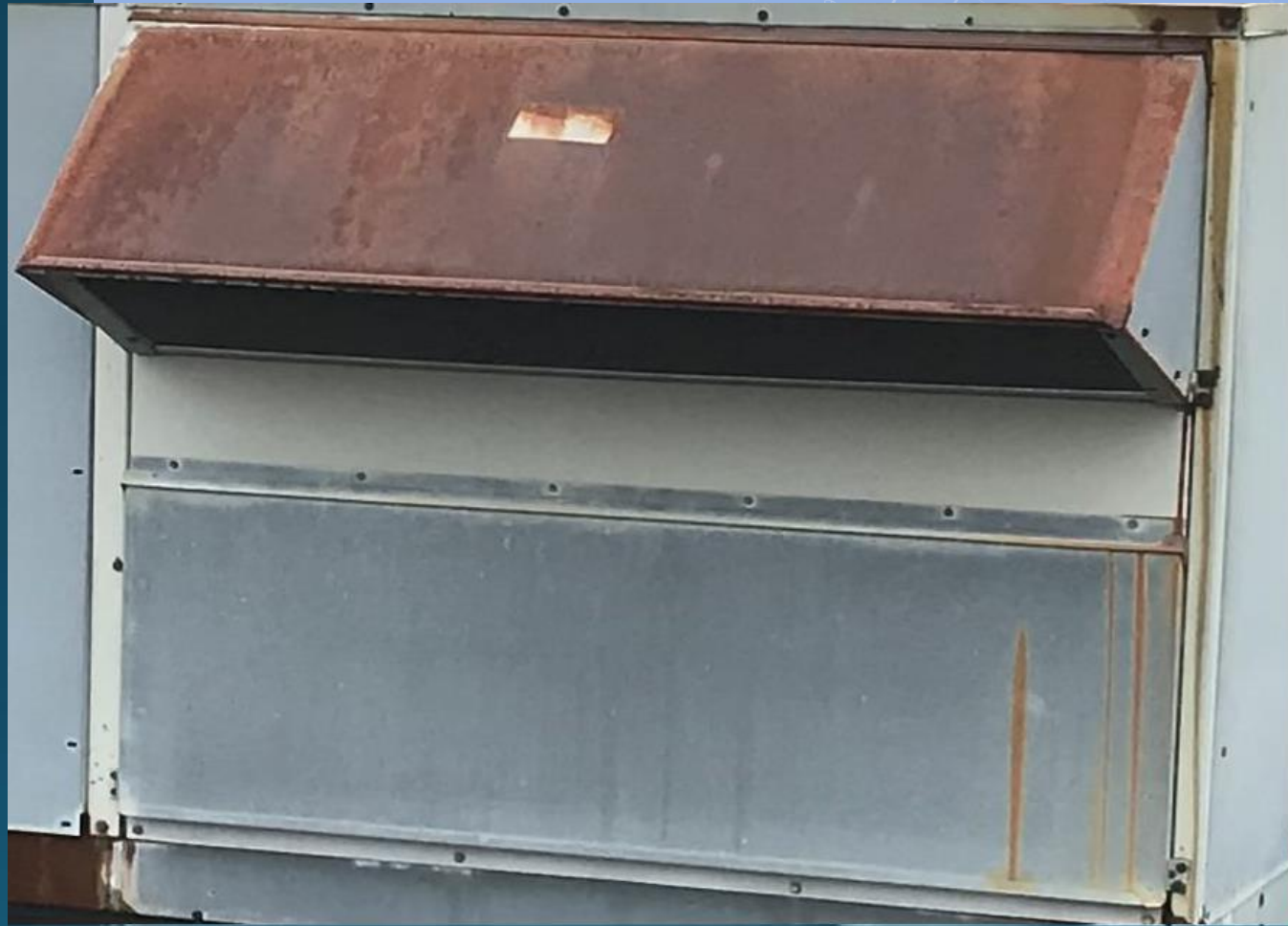
One of 3 Main HVAC units for building. All 1984. Cooling operational, heating disabled. Beyond 20 yr service life at 39 yrs. old.
