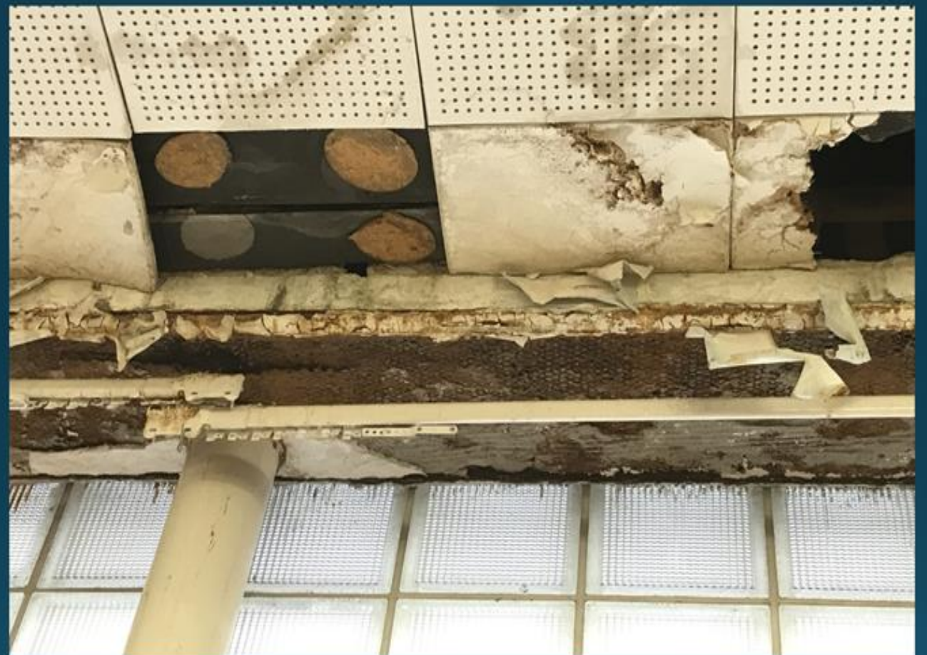
Extensive damage to Third Floor ceiling/window soffit area from prior roof drain leakage. Also note, asbestos around outside edge of all glass block walls/windows.
