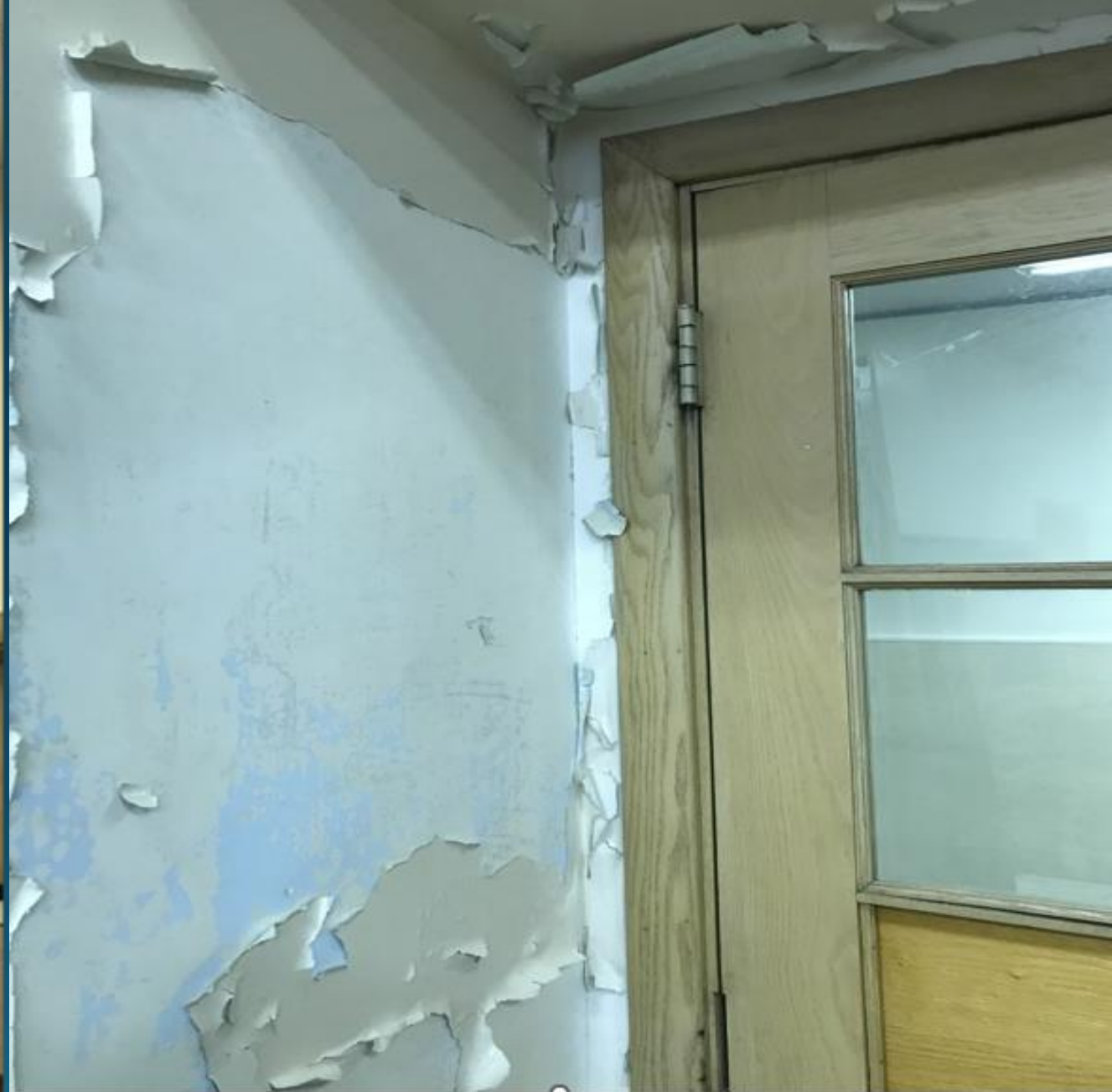
Third floor paint damage.
